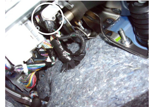
Solder White wire onto Black ground wire. Solder Yellow wire onto Light Red wire on the clutch switch.
